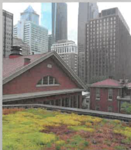
A green roof on Philadelphia's Friends Center captures runoff and insulates the building while adding natural beauty to the cityscape.
